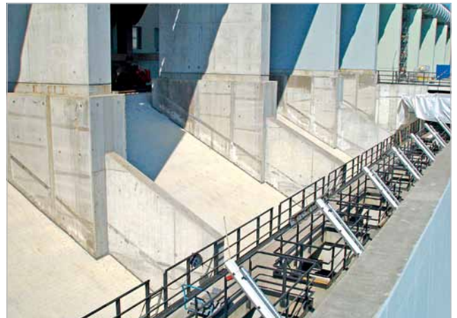
Coke wharf protected with KALCERAM-K on the sliding surface, with KALSICA-N in the zone of high wear and with KALMETALL-C in the area of impact stress
