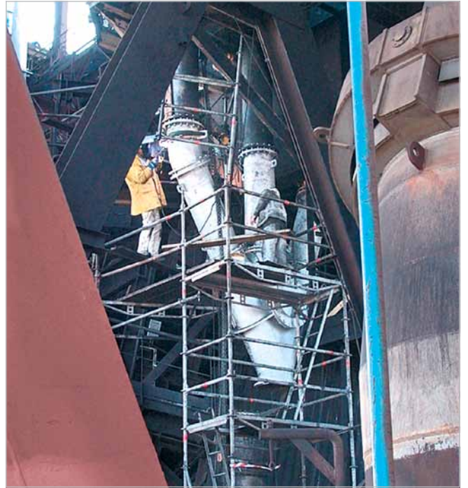
Pressure equalizing pipe set up near a blast furnace; the base metal has a thickness of 30 mm, the thickness of KALMETALL-W 100 hard overlay welding measures 6 mm; 450 mm diameter
