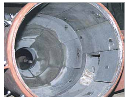
Cyclone used in a soil decontamination system – effectively protected with KALMETALL-C
