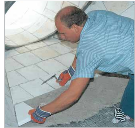
KALCOR lining of a hopper in the sinter dust collector of a steel mill
