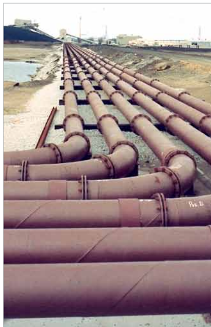
Worldwide ash removal pipes lined with ABRESIST reach lifetimes of more than 30 years. This US power plant operates more than 10,000 meters of 294 mm ID pipes.
