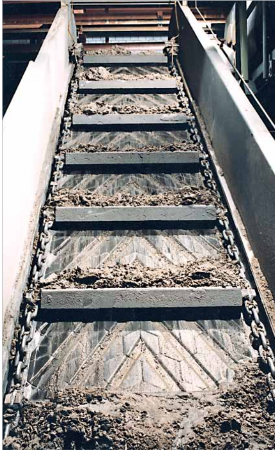
Chain conveyor for wet ash removal in a power plant. Drains cast into the lining reduce the undesired carrying of water to the discharge zone thereby lowering the water consumption rate.
