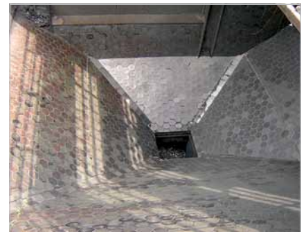
Coke bunker in the iron and steel industry
