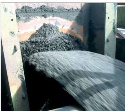
KERFALEX lining of a bin set up in a bulk material handling plant
