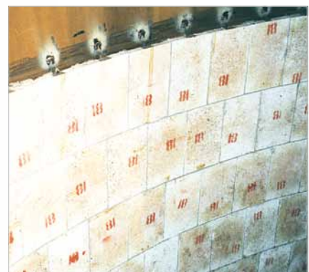
High temperature wear protection in a dedusting cyclone of a blast furnace plant in Europe
